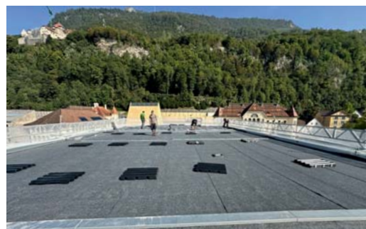
The solar panel unit on the roof of Äule House commenced operating at the end of October.
