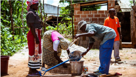
The ORATTA project supported the expansion of drinking water facilities in Mozambique in 2023
